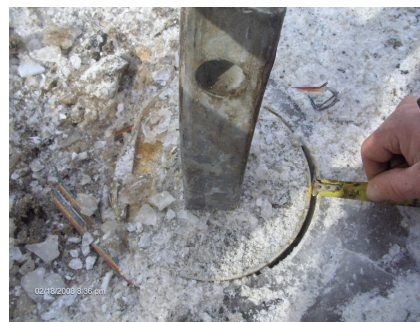
Figure.13. FRP-G-HSP with external grout separation between the FRP tube & external grout during lateral testing
