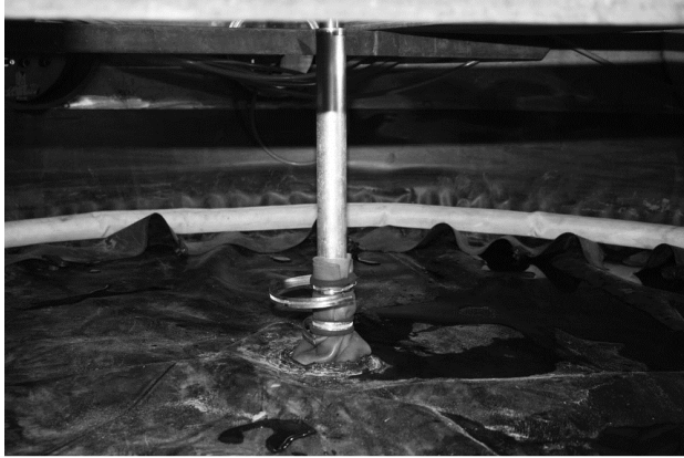
Figure 4. The membrane placed on the soil surface and secured around the pile by hose clips and against the side of the tank by a fire hose.
