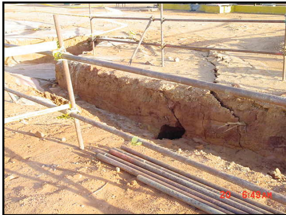
Figure 14. Crack and settlement in the area of collapse of the soils after intense rains.
