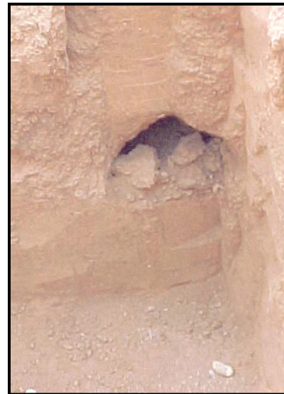
Figure 4. Natural cavity in collapsible soils found during an excavation.
