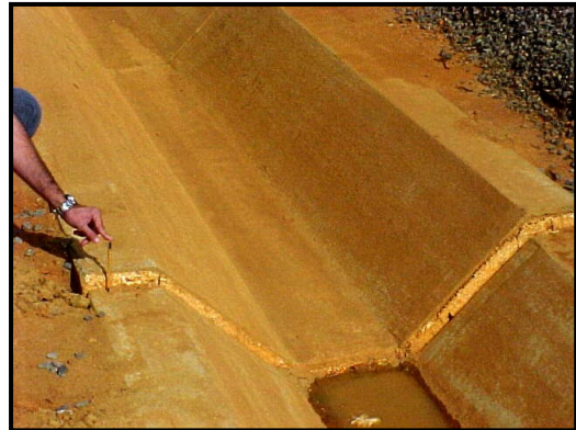
Figure 15. Settlement of 5 cm induced by the collapse of the underlying soil
