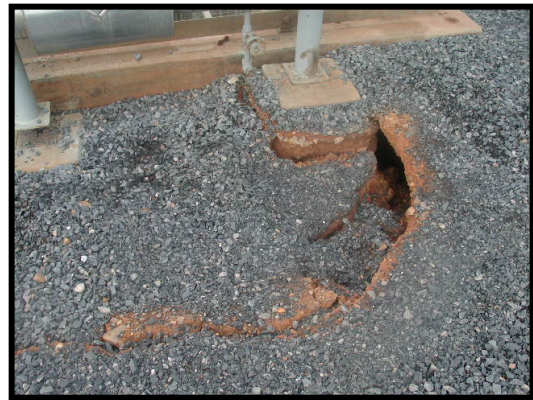
Figure 16. Settlement of an area close to a water structure with an opening cavity.
