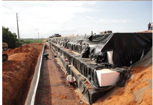
Figure 14. Use of EPS blocks as lightweight fill material: a) installation of the blocks b) cross section showing blocks and protective cover (BR-101).
