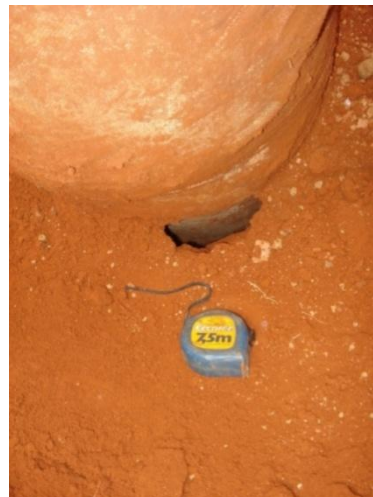
Figure 8. Gap between encased column and borehole due to the column execution process.
