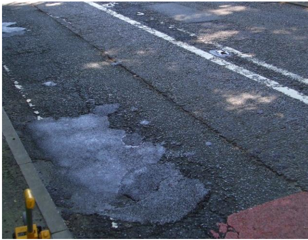
Figure 9. Localised failure and cracking through a section of the scheme
