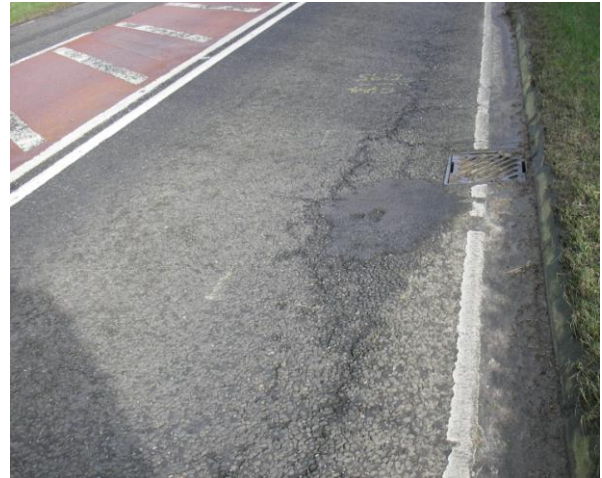
Figure 4. Wheeltrack cracking through a section of the scheme
