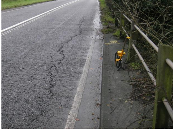
Figure 1. Wheeltrack cracking through a section of the scheme
