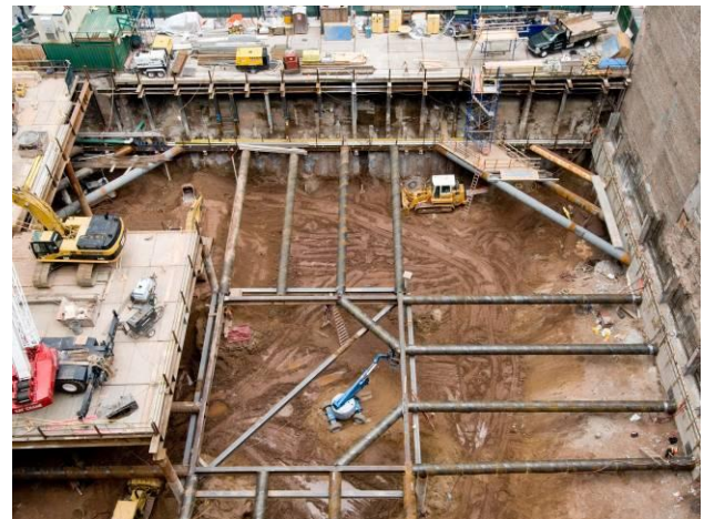
Figure 6. Aerial view of the Transit Center site, October 2009 (facing north from the Corbin Building).
