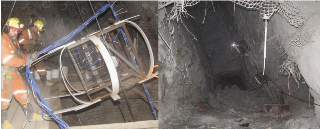
Figure 1. Cages were lowered down the Alimak raise at Williams mine (left), and anchored in the undercut (right)
