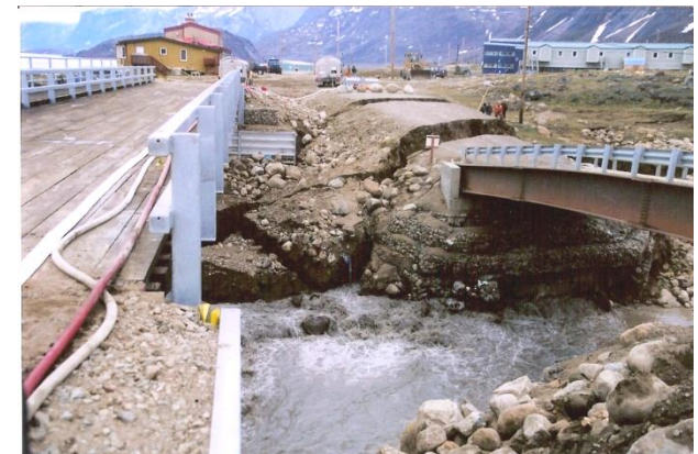
Photograph 4: Failure of North Approach Fill
