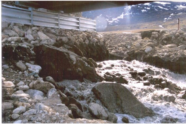
Photograph 6: Water Flowing Underside of Bridge Foundation
