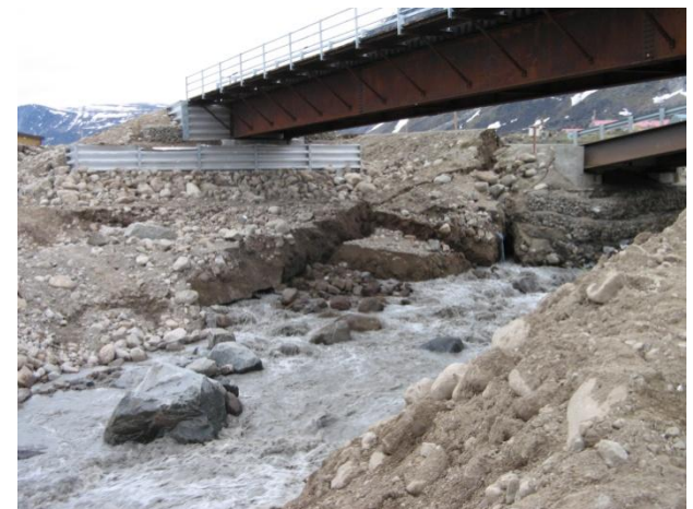
Photograph 5: Failure of North Bank
