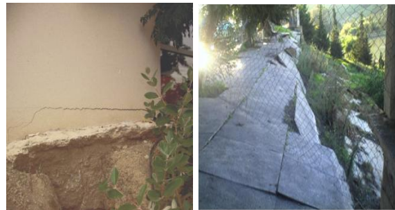
Figure1. Cracks on structure and walking path degradation due to soil movement within Marley soils (West of Algiers)
