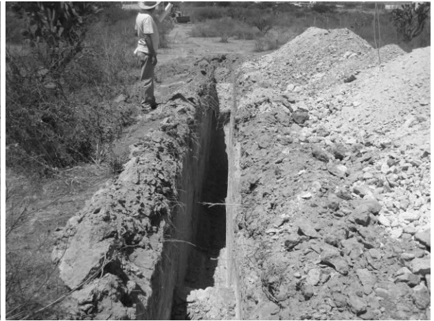
Figure 17. Excavated trench for carrying out a direct exploration in the stretch where the interpretation of the anomalies of resistivity presents ambiguities.
