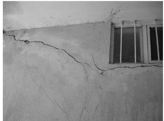
Figure 4. Caused damage to a bearing wall by differential settlement
