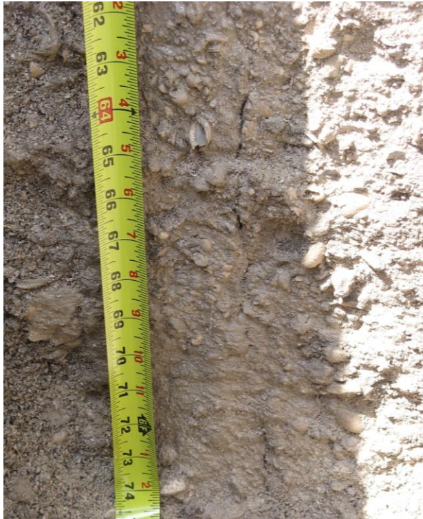
Figure 3. Wall cracking observed in a test pit.
