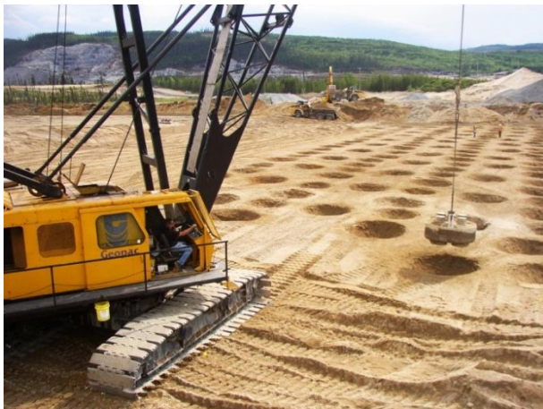
Figure 2. 125 ton capacity crane and 15 tonne tamper used for the Peribonka Dam (Québec) foundation densification.
