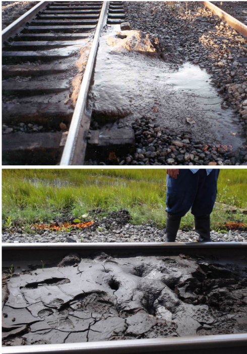
Figure 2: Examples of silt/clay plumes developed within the railway embankment, day lighting at the surface of the ballast.
