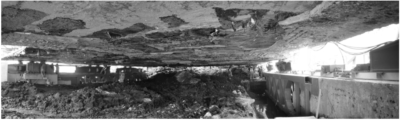
Figure 10. Panoramic view under the house foundation being supported by the hydraulic jacks prior to its moving
