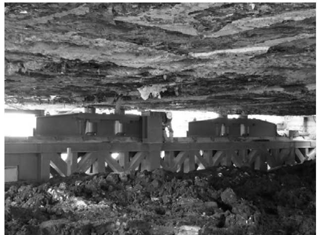
Figure 7. View of the truss placed between diaphragm walls after the hydraulic jacks had been positioned
