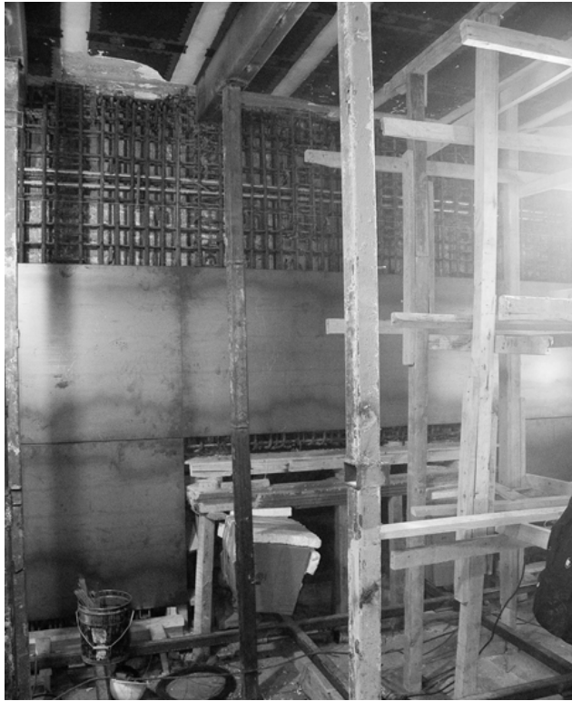
Figure 4. Strengthening of the house with reinforced concrete walls (Courtesy of Fondo Hexa)
