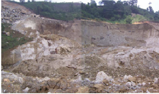
Figure 3. Remnant escarpment of failure seen from the right bank. From RVO y Cía. (2006)
