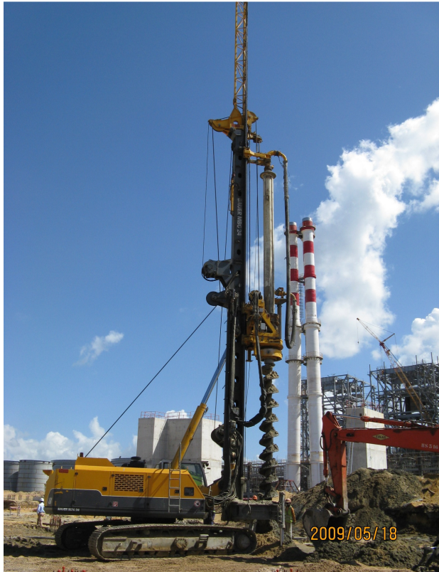
Figure 10. Typical CFA Piling Rig
