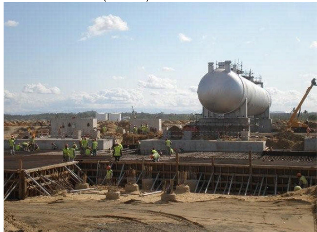
Figure 1. Autoclave Installed at the Process Plant
