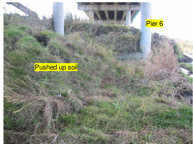
Figure 3. Soil pushed up near Pier 6 (looking south)
