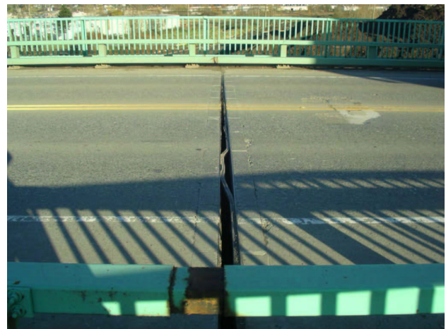
Figure 7. Uneven displacement of expansion joint at Pier 6, and traffic rail pulled apart at the west side (foreground)
