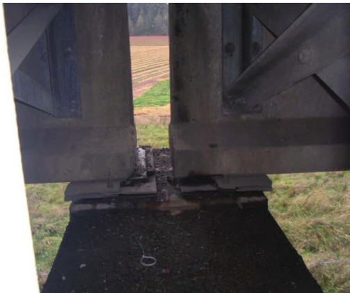
Figure 6. Displaced girder at Pier 6 (looking west)
