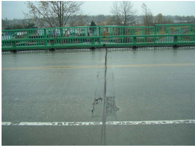
Figure 8. Uneven displacement of expansion joint at Pier 8, and handrail pulled apart at the east side (far side)
