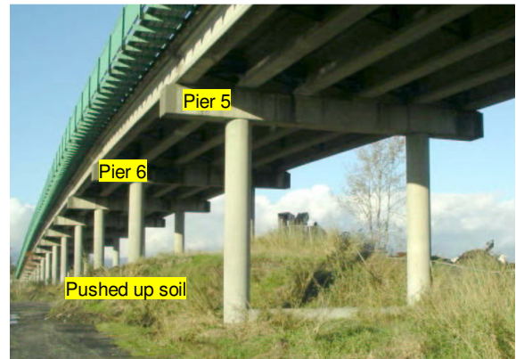
Figure 2. Soil pushed up between Piers 5 and 6 (looking north)
