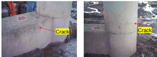
Figure 5. Cracks in pile cap beam and column at Pier 6
