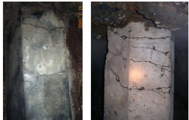
Figure 10. Cracks in precast piles at Pier 5 and Pier 6 on the west side
